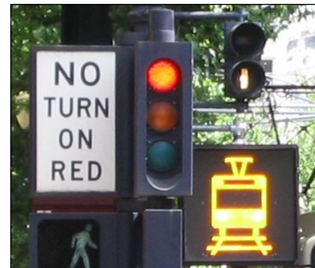
Portland, Oregon - Typical rail transit signal and roadway traffic signal shown together for mixed traffic operations
