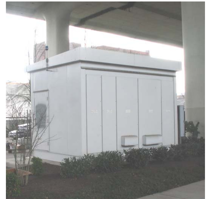
Portland, Oregon—Traction Power Substation
